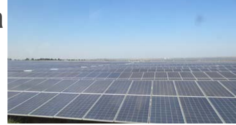
Pavagada Solar Park– Sea of Glass
